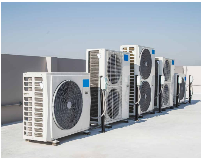
Rooftop heat pumps
