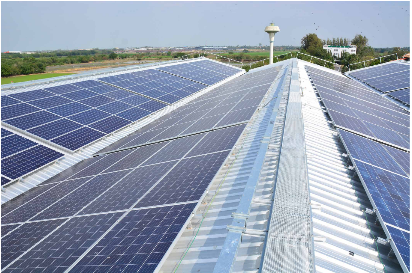
Rooftop solar photovoltaic (PV) system
