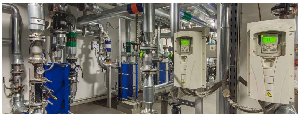
Variable speed drives
