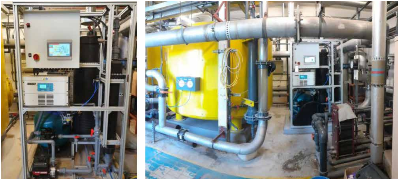
Backwash water recovery system
